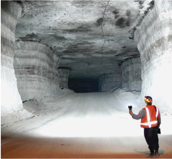
Fig. 6. Stable pillars in a limestone mine at a depth of cover of 275 m. Slightly concave pillar ribs formed as a result of minor spalling of the hard, brittle rock.
