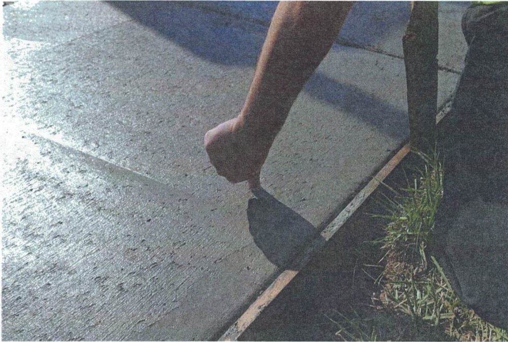
Ready for final finishing operations – thumb makes an easy impression in the concrete about a half an inch.
