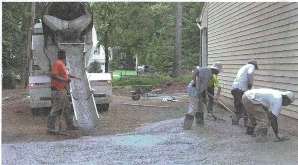
Slump that exceeds 5 inches may be easier to place but should never be used for slabs unless the slump is achieved using a high range water reducer. High slump concrete without high range water reducers can have excessive and prolonged bleeding, a tendency to segregate (separation of paste and stone), lower strengths, longer set times, and a higher likelihood for scaling.
