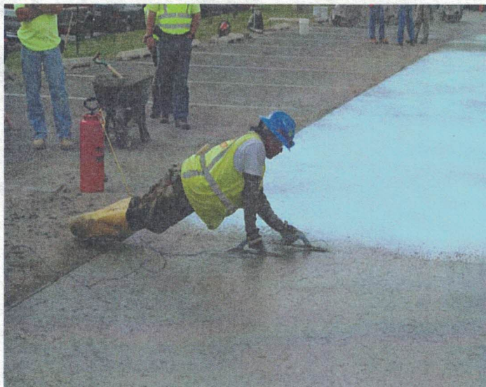
Too late – concrete has set where final finishing will be extremely difficult
