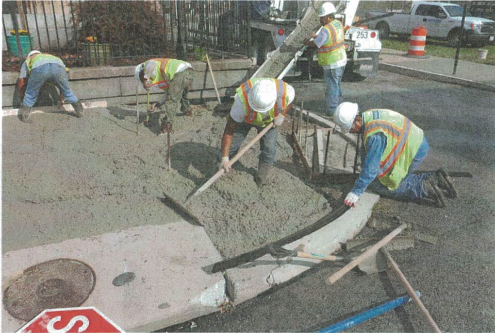
Properly proportioned concrete with a slump around 3 to 5 inches is relatively easy to place and finish. The mixture holds together well.
