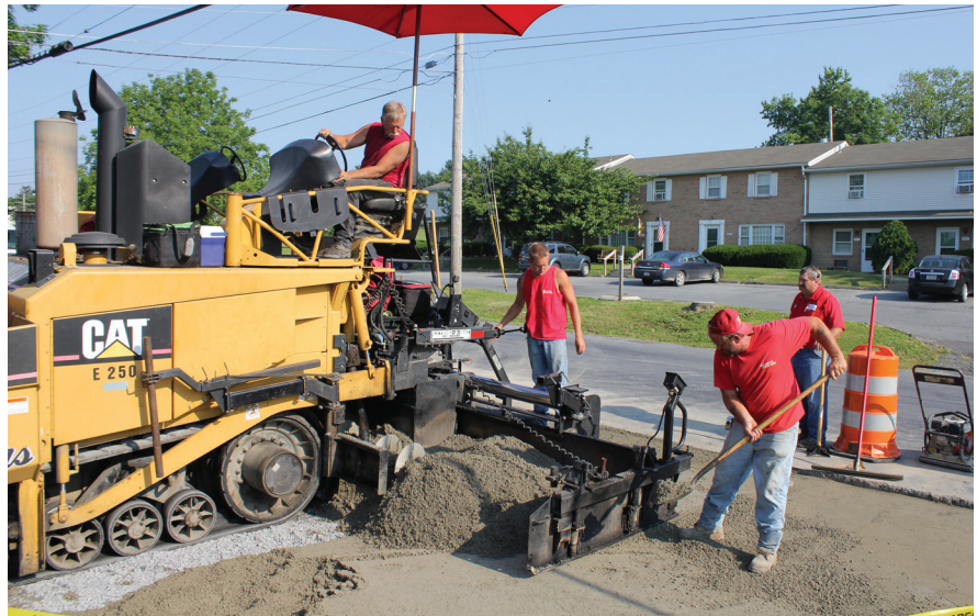
Upper Nazareth Township in Northampton County served as a test site for roller-compacted concrete, a low-cost paving option. The material was applied to a 420-foot section of road that has been in use for about two months. “It looks as good as the day we finished it,” an official says. “We’ve had absolutely no complaints.” (Photo courtesy of Sean Dooley, Keystone Consulting Engineers.)
